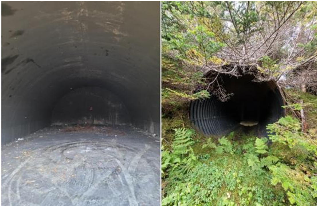
Figure D2-3.2-1 Relic Military Bunkers Which Could Have Potential as Bat Roost Sites.
