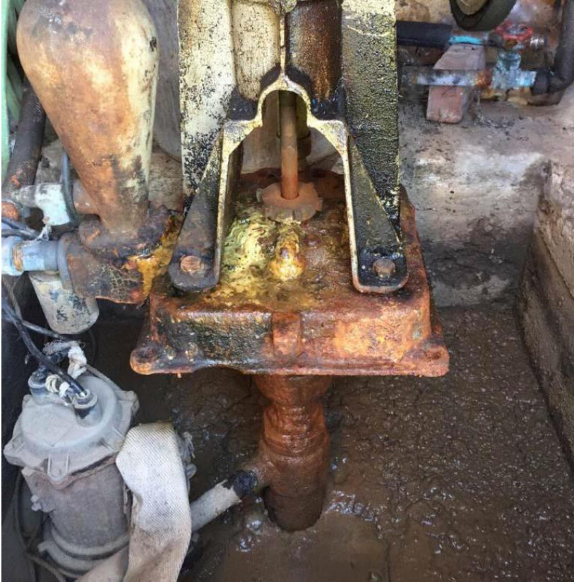
Photograph 3: Well 12 illustrating pump mounted directly on well casing.
