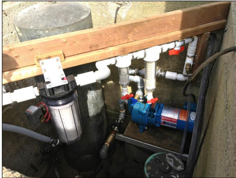
PHOTO 2: Particle Filter System (as observed by AECOM on 14-August-2017 & 28-August-2017)
