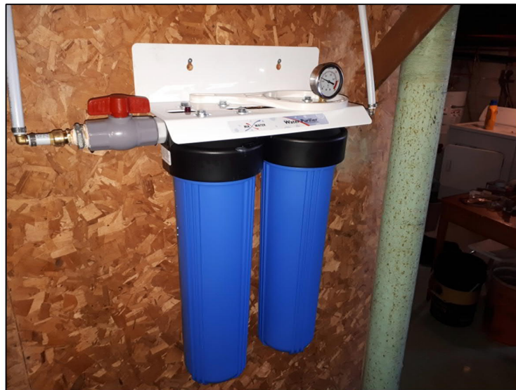
PHOTO 3: Water Filtration System on Distribution (as observed on 7-November-2017)
