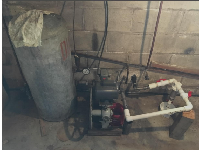
PHOTO 2: Well Pump & Sediment Filter System (as observed on 7-November-2017)
