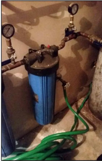
PHOTO 2: Particle Filter System (as on 2-February-2017). Opposing side of wall from recent photograph. (Presence unconfirmed during 2-August-2017 site visit)
