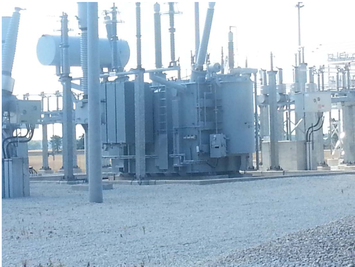
Photograph #2 of the Ripley Substation
