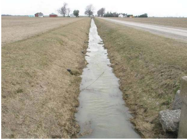
Field Plate 51.25: View southeast along Collector Line on Merlin Road at wide ditching – no potential.
