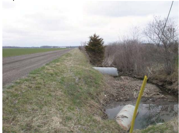
Field Plate 53.26: View northeast along Collector Line on Stefina Line at disturbed roadbed and ditching – no potential.
