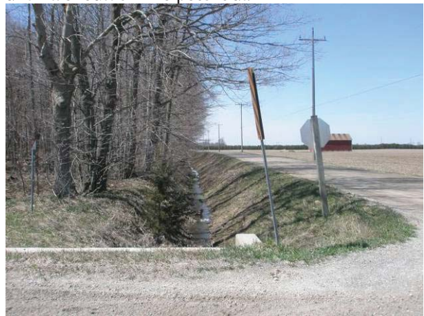
Field Plate 52.16: View northwest along Collector Line on Lagoon Road, west side, at wide deep ditching in ROW – no potential.
