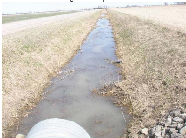
Field Plate 51.36: View north along Collector Line on Oak Road, east side, towards Pollard Line at roadbed and wide ditching.
