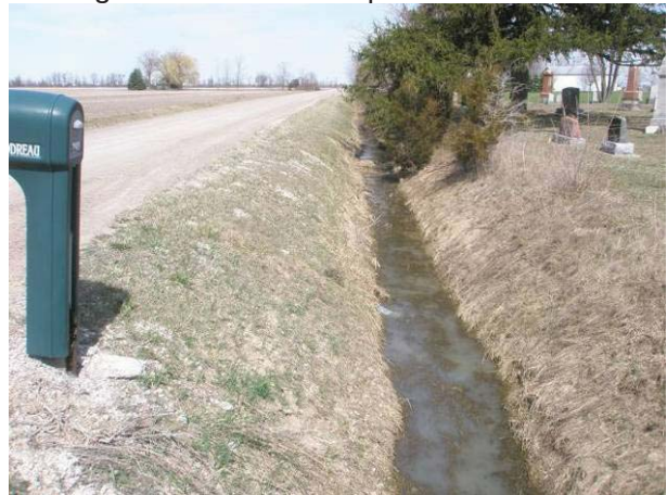
Field Plate 51.48: View northeast along Collector Line on Coatsworth at Rosedale Line, west side, at roadbed and ditching in ROW with no potential.
