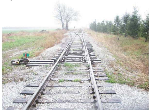
Field Plate 52.22: View southeast along rail line adjacent Fargo Road at disturbance.
