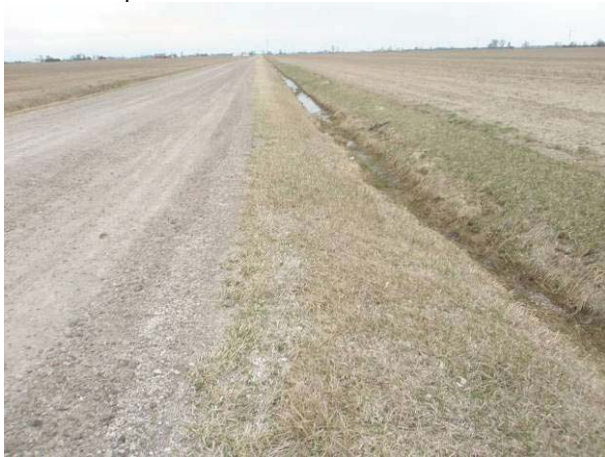
Field Plate 51.3: View south along Collector Line on Irwin Road, west side, at raised roadbed and ditch – no potential.
