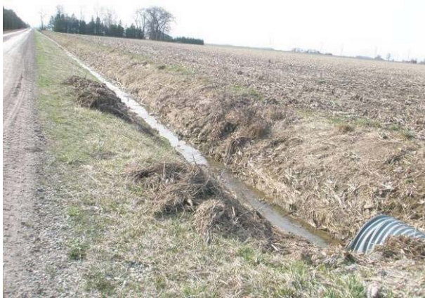
Field Plate 51.27: View southwest along Collector Line on Morris Line, south side, at Cooper Road intersection at disturbed roadbed and ditching – no pot'l.
