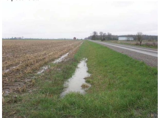
Field Plate 53.8: View northeast along Collector Line on Welch Line at raised roadbed, fill slope and ditching – no potential.
