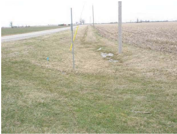
Field Plate 51.7: View north along Collector Line on Port Road, east side, at roadbed and ditching in ROW – no potential.
