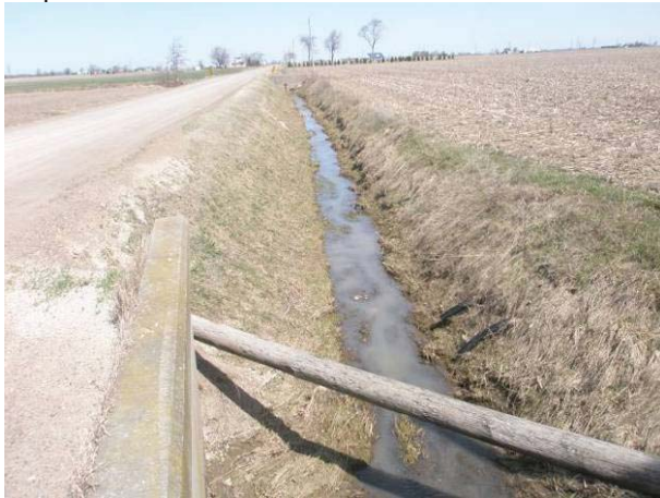
Field Plate 51.39: View north along Collector Line on Oak Road from Gray Line at disturbed ROW with no potential.
