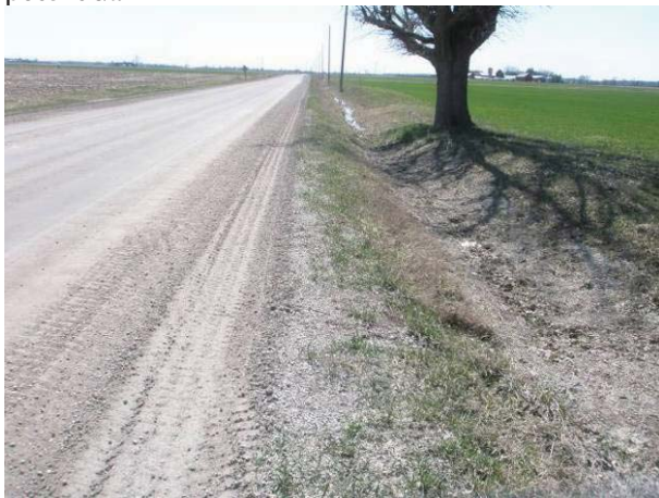
Field Plate 52.15: View southwest along Collector Line on Horton Line at narrow ROW with ditching and no potential.
