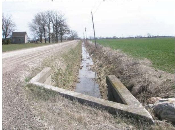
Field Plate 51.42: View east along Collector Line on Gray Line, south side, at ditching in ROW – no potential.
