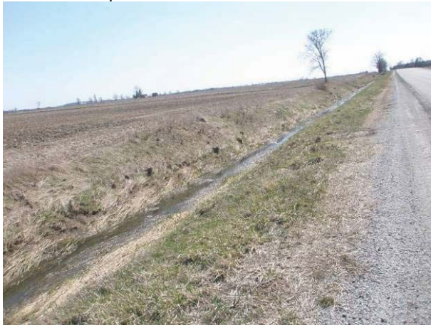
Field Plate 52.21: View northwest along Collector Line on Fargo Road at disturbed roadbed and ditching – no potential.
