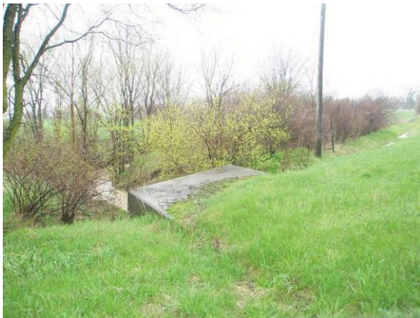
Field Plate 52.63: View west across Collector Line on Shewburg Road at fill, ditching and low/wet areas adjacent to roadway.
