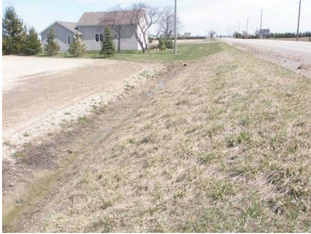
Field Plate 51.45: View northeast along former Collector Line route on Middle Line, north side, at wide ditching in ROW – no potential.
