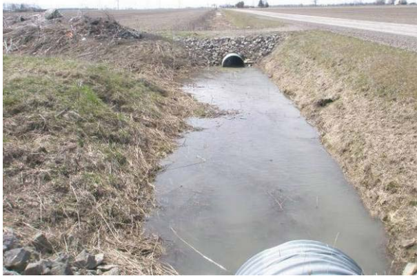
Field Plate 51.37: View south along Collector Line on Oak Road, east side, at raised roadbed and ditching – no potential.
