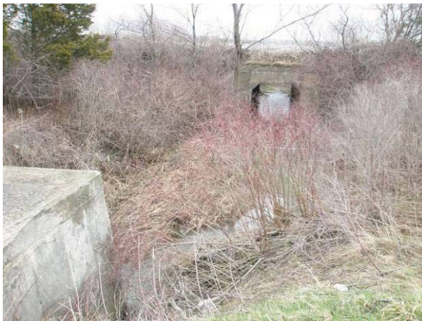
Field Plate 52.51: View northeast along Collector Line on Knights Line at substantial ditching adjacent roadway.
