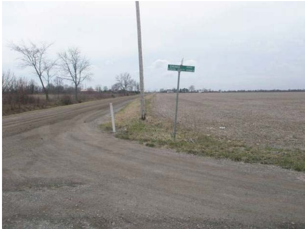
Field Plate 51.19: View southwest along Collector Line on Seventh Line, north side, at raised roadbed and ditching to limit of ROW (pole) – no potential.
