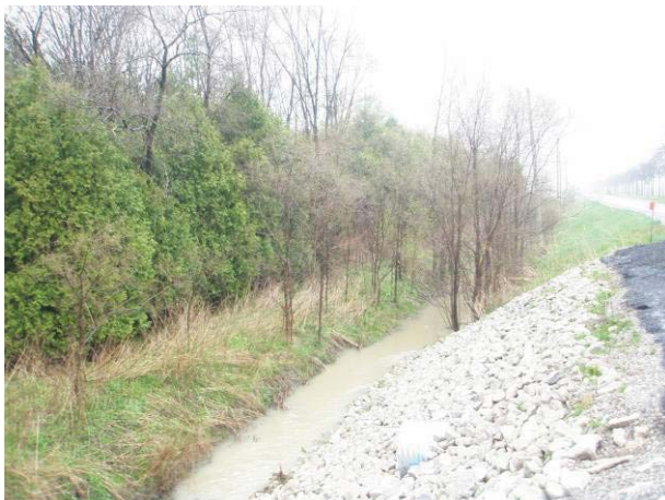
Field Plate 52.29: View northeast along Collector Line on Boundary Line, south side, at raised roadbed ditch in ROW – no potential.
