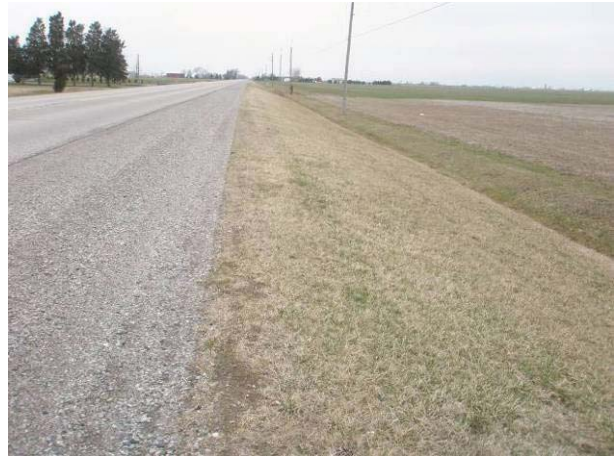
Field Plate 51.2: View west-northwest along Collector Line on north-side Middle Line at raised roadbed and ditch – no potential.
