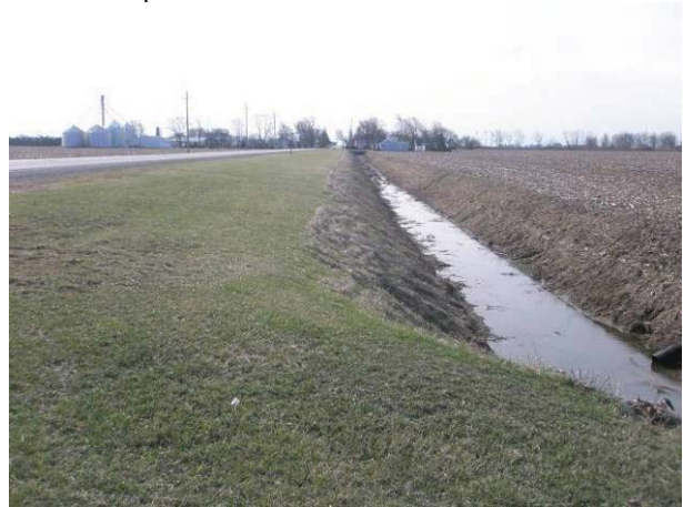
Field Plate 51.4: View east along north side Pollard Line at wide ditching typical of ROW with no potential.
