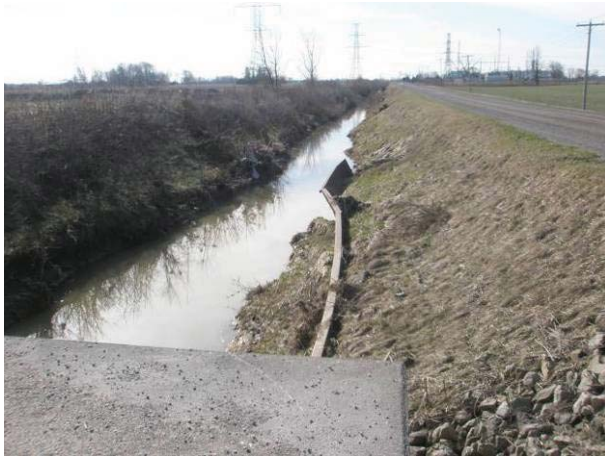
Field Plate 51.55: View southeast along Collector Line on Dillon Line, east side, at wide ditching in ROW – no potential.
