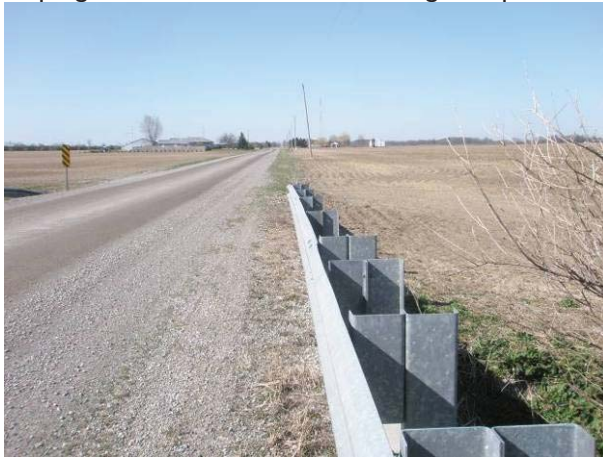
Field Plate 51.63: View southwest along Collector Line on Ninth Line, north side, at raised roadbed and fill slope to limit of ROW with no potential.
