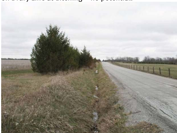
Field Plate 52.47: View southeast along Collector Line on Harwich Road at roadbed and ditching – no potential.
