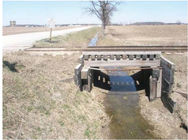
Field Plate 52.20: View northeast along Collector Line on Horton Line, east side, at wide ditching in ROW – no potential.
