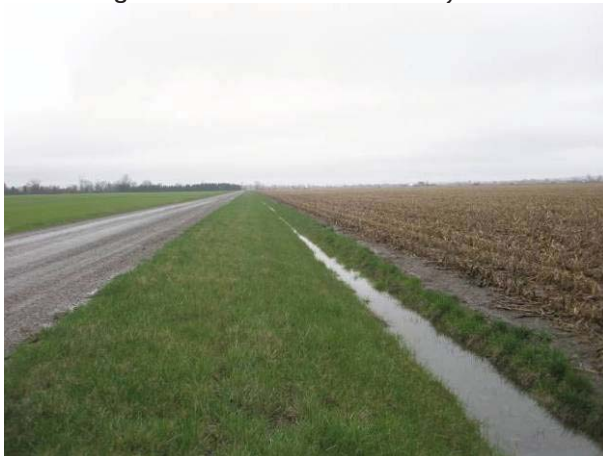
Field Plate 53.13: View NE along Collector Line on Coffell Line at disturbed roadway and ditching. Spot testing was performed at areas with perceived pot'l.
